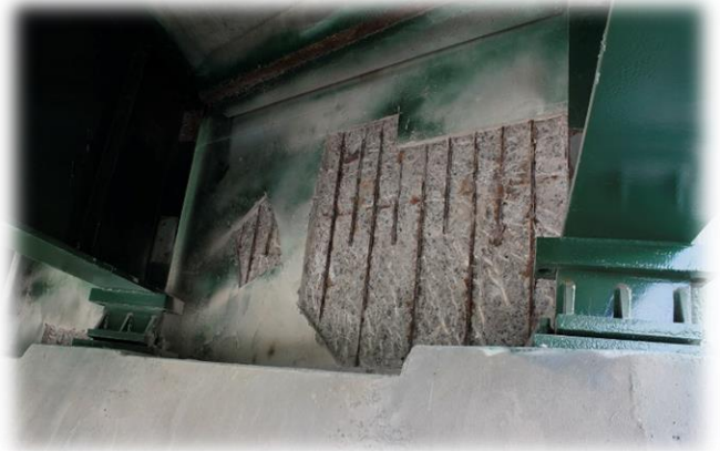
Delaminated Concrete Removed from Backwall
